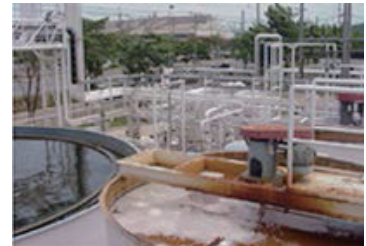
General effluent treatment facilities
