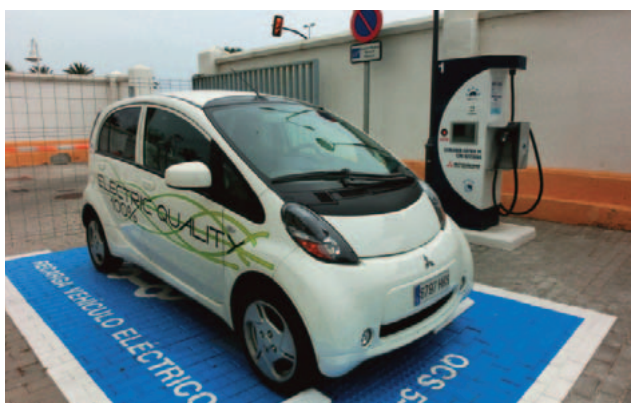
Rapid charging stations were installed in the city of Málaga
