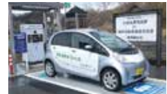
Quick charging station installed in a roadside station in Yamagata Prefecture
